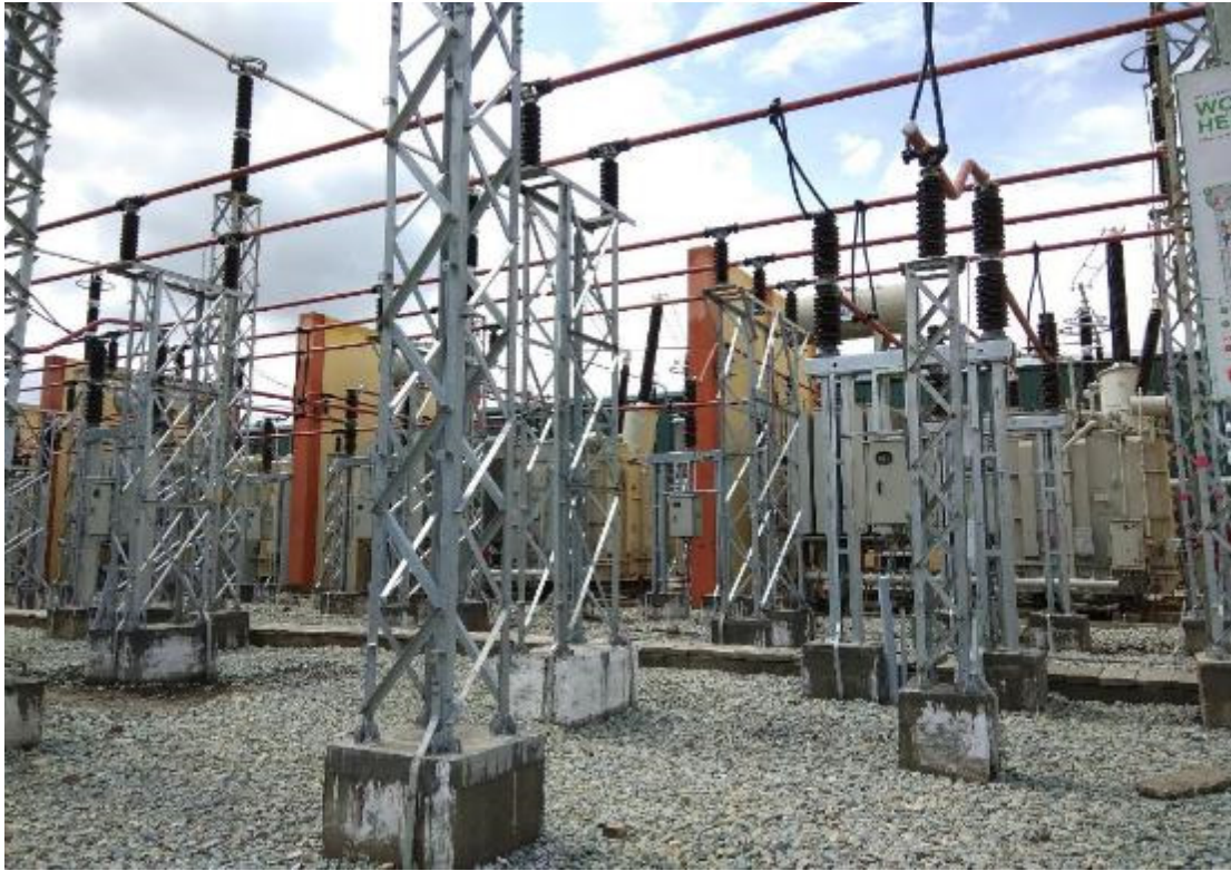
Inter – Connecting Sub – station yard
