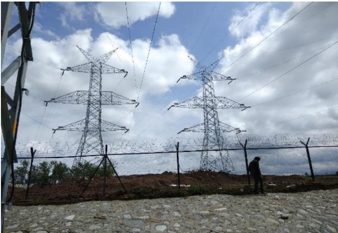
220 kV outgoing transmission lines
