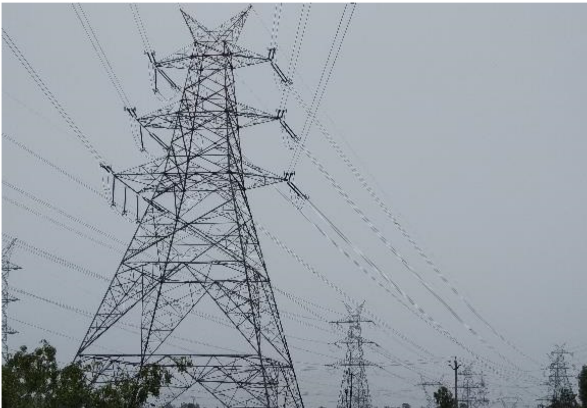
Jalandhar – Samba 400 kV D/C Powerline crossing
